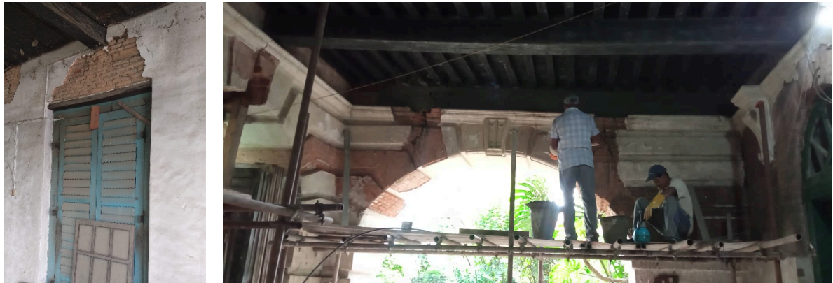
Figure 14. Photographs of the cracks in the openings and the arches after the 2015 earthquake
